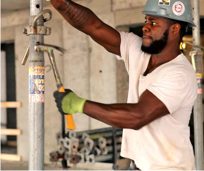
After going through the New Jersey Reentry Corporation’s program, Jamar was hired as a construction laborer. His current construction project is a high rise residential building in Jersey City.
